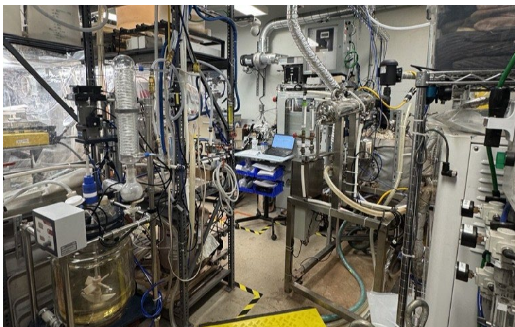
Figure 4: Pilot plant setup at the Boucherville facility
