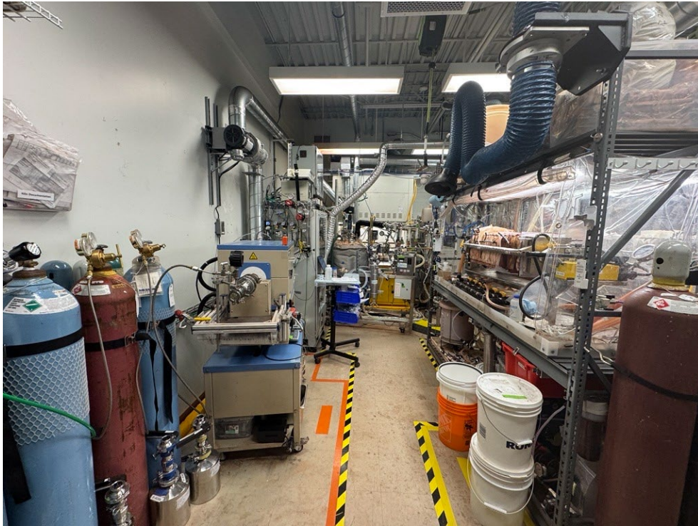
Figure 3: Pilot plant setup at the Boucherville facility
