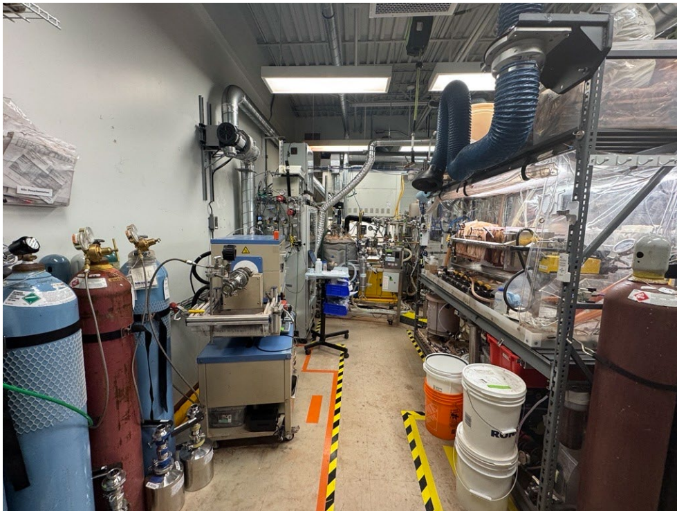
Figure 3: Pilot plant setup at the Boucherville facility
